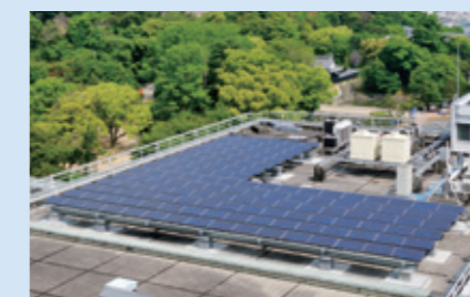
Solar panels (NTT West, Kochi Branch)
