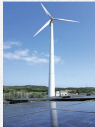
NTT FACILITIES' hybrid wind/solar power station on the island of Kumejima
